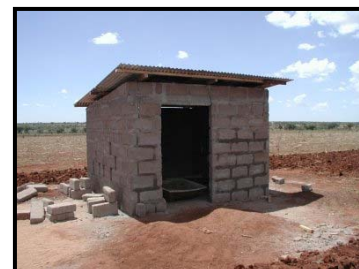
New Pump House
